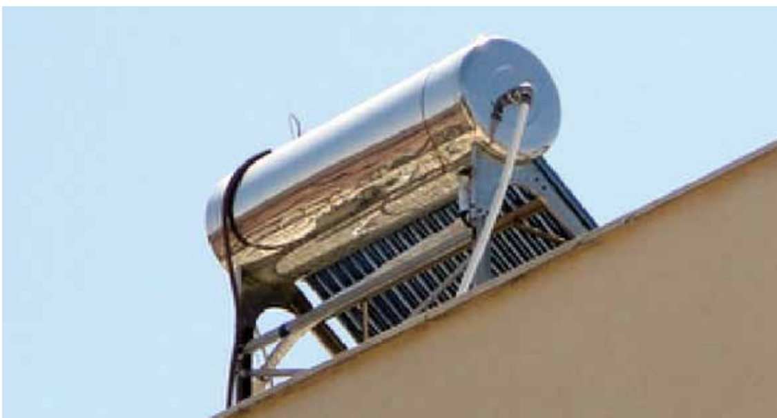
Figure 6: A solar water heater on the roof of the building of a Jordanian private hospital
