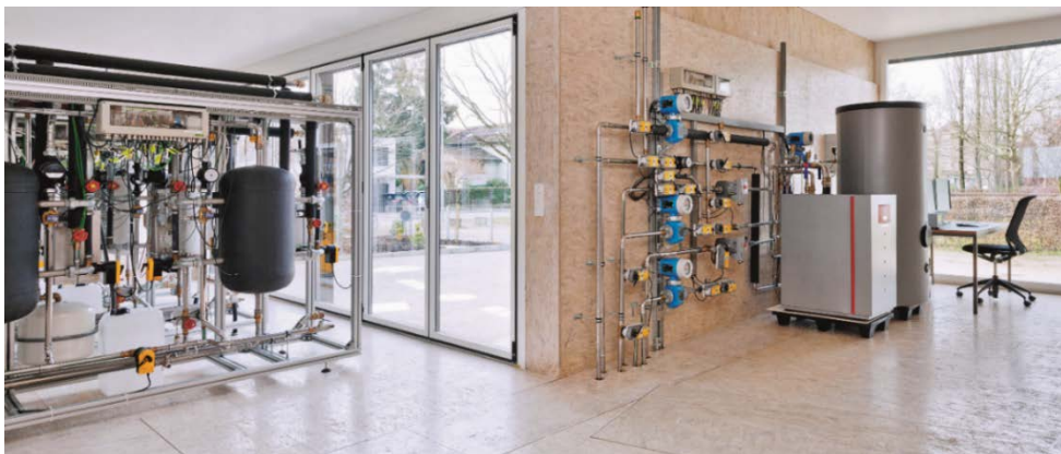
Figure 2. Second stage of the thermodynamic core (left). Heat pump and domestic hot water storage (right).
